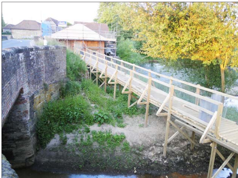
Progress with the new boardwalk, part of the development at Coultershaw. Visitors will be able to use the boardwalk to access the former lock on the Rother Navigation that now has a footpath laid through it. (Martin Snow)
