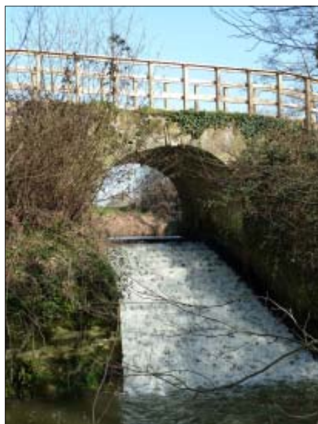
Grade II listed Stream Bridge in deepest Sussex, north of Chiddingly, close to the village of Gun Hill, see the article on page 10. ( Malcolm Dawes )
