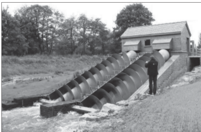
A typical archimedean screw installation used for power generation
