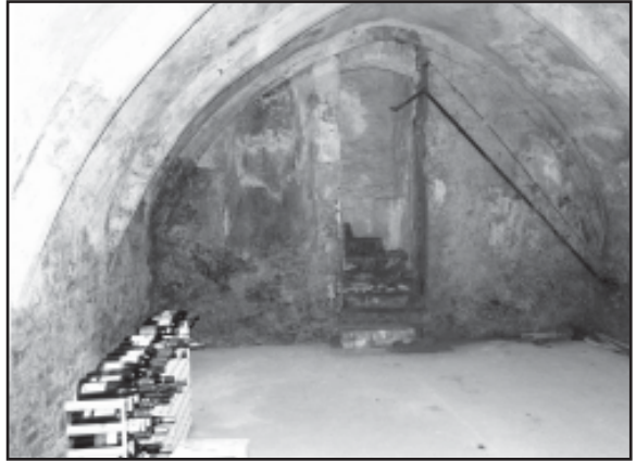
One of Winchelsea's vaulted cellars, still being used to store wine. The blocked steps went to the property above - an unusual feature for Winchelsea. ( Martin Snow )
