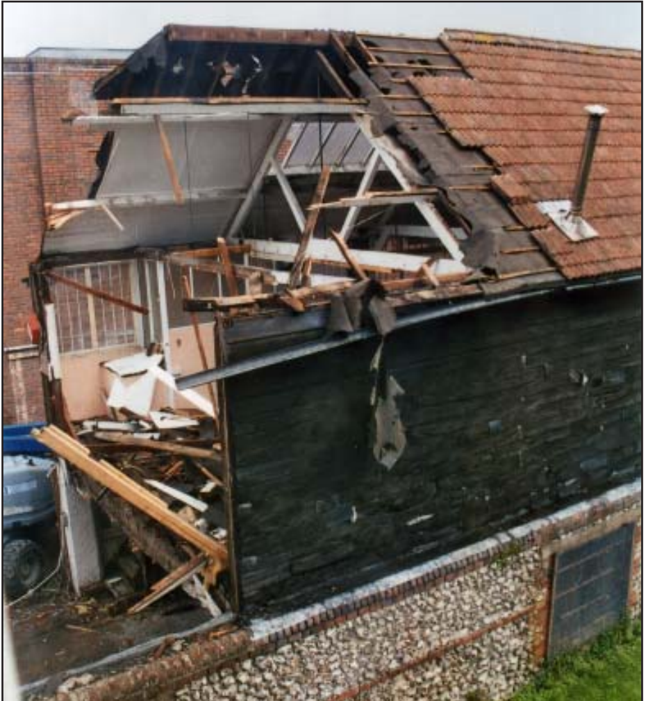
Demolition in progress on the former printing works in St John's Street, Chichester
