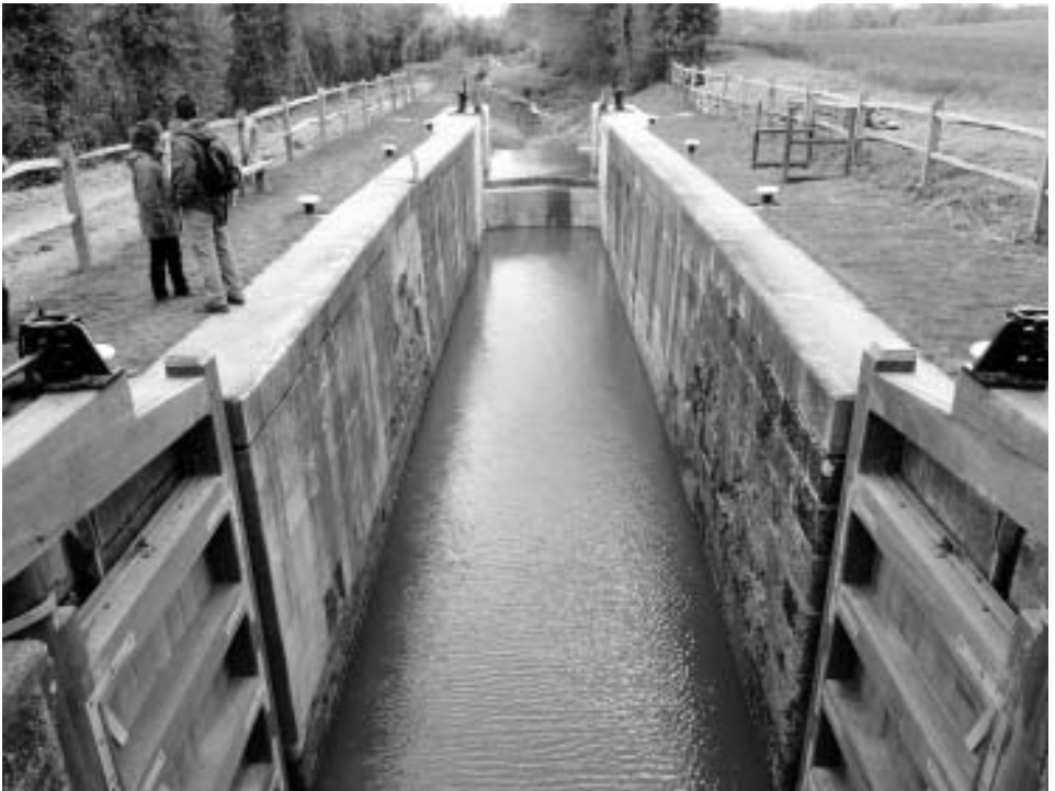
Devil's Hole Lock, newly restored by the Wey and Arun Canal Trust.
